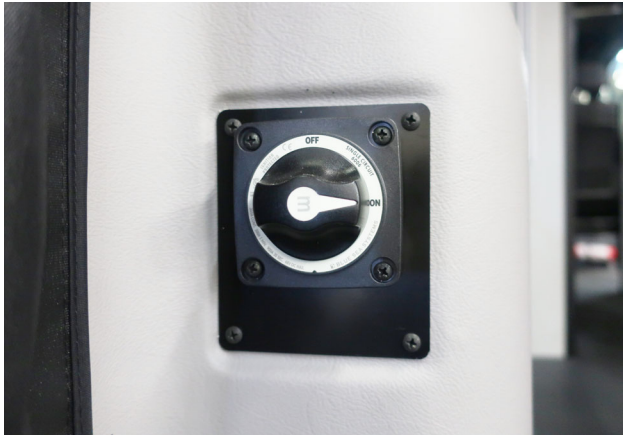
Inverter/charger disconnect switch. (Located behind the driver's side rear door) -Typical View
