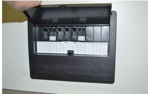
120-Volt Circuit Breakers -Typical View
