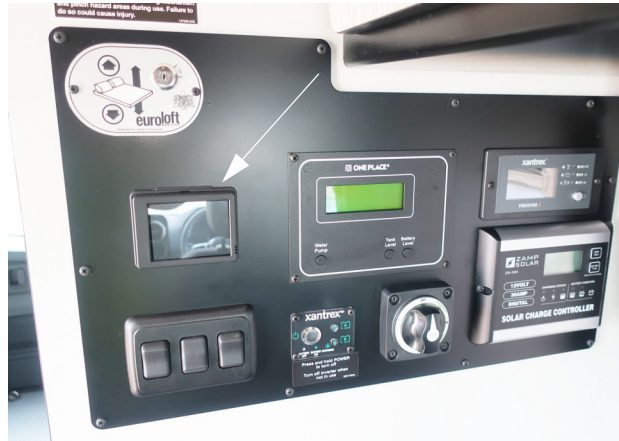
LCD Panel (Located near monitor panel) -Typical View
