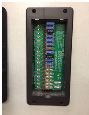
House 12-Volt Fuses -Typical View
