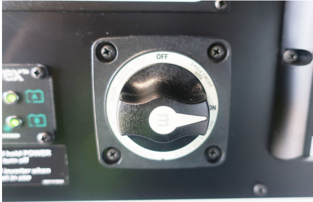
Solar Power Disconnect Switch (Located near monitor panel) -Typical View
