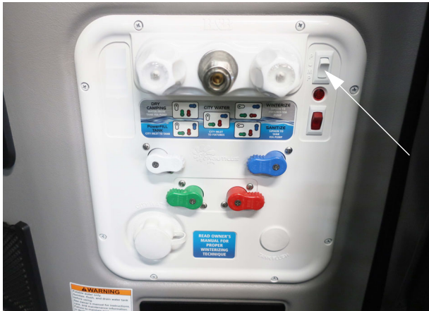
Water pump switch location on Water Center Panel -Typical view
